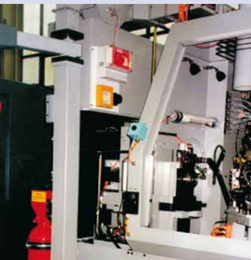
Fire suppression units
